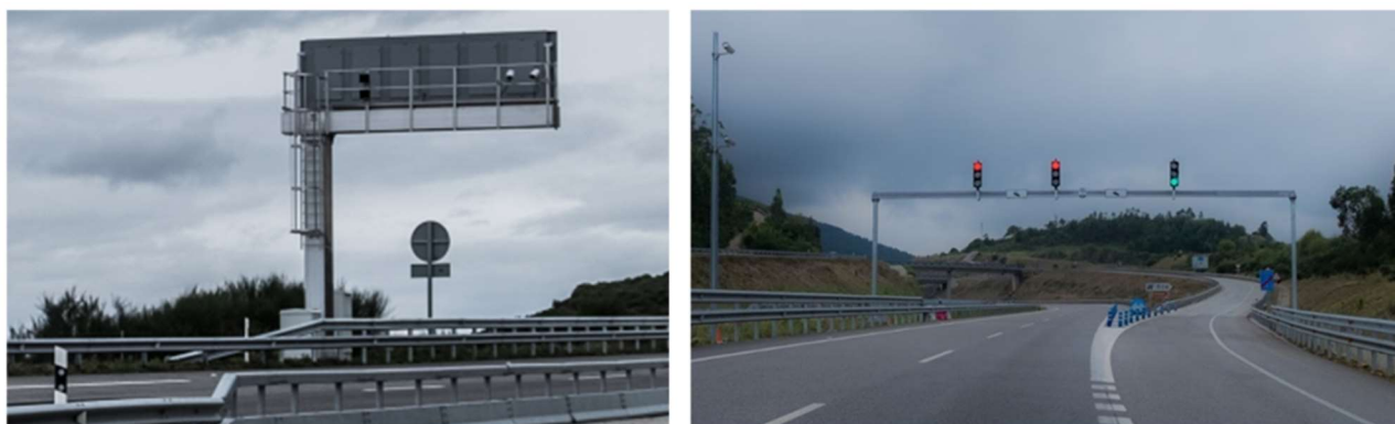
Figure 9. Variable Message Sign and traffic lights with red light cameras. A-8 Motorway. Alto del Fiouco (Lugo). Spain
