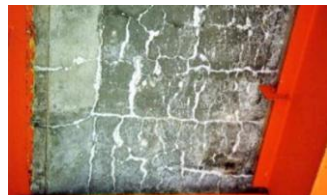
SLAB (Two-Way Cracks and Efflorescence)
