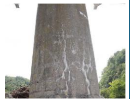
PIER (Cracks and Efflorescence)
