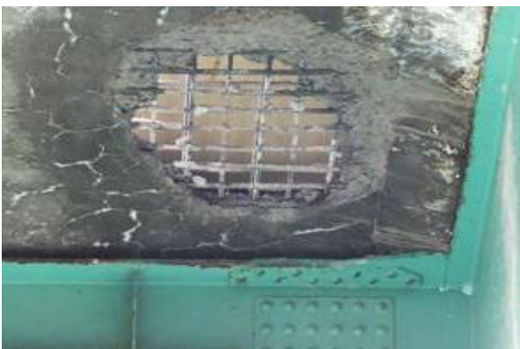
Deck slab collapse
