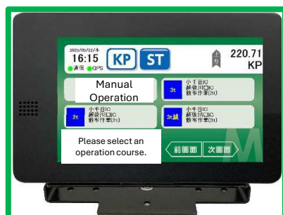
Integrated control panel
