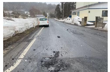
Early detection of potholes during the snowmelt season
