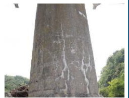
PIER (Cracks and Efflorescence)
