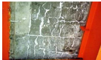
SLAB (Two-Way Cracks and Efflorescence)
