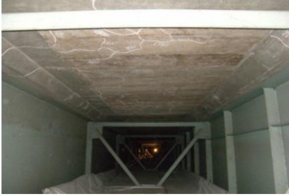
Occurrence of cracking
