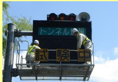
Inspection for message sign board
