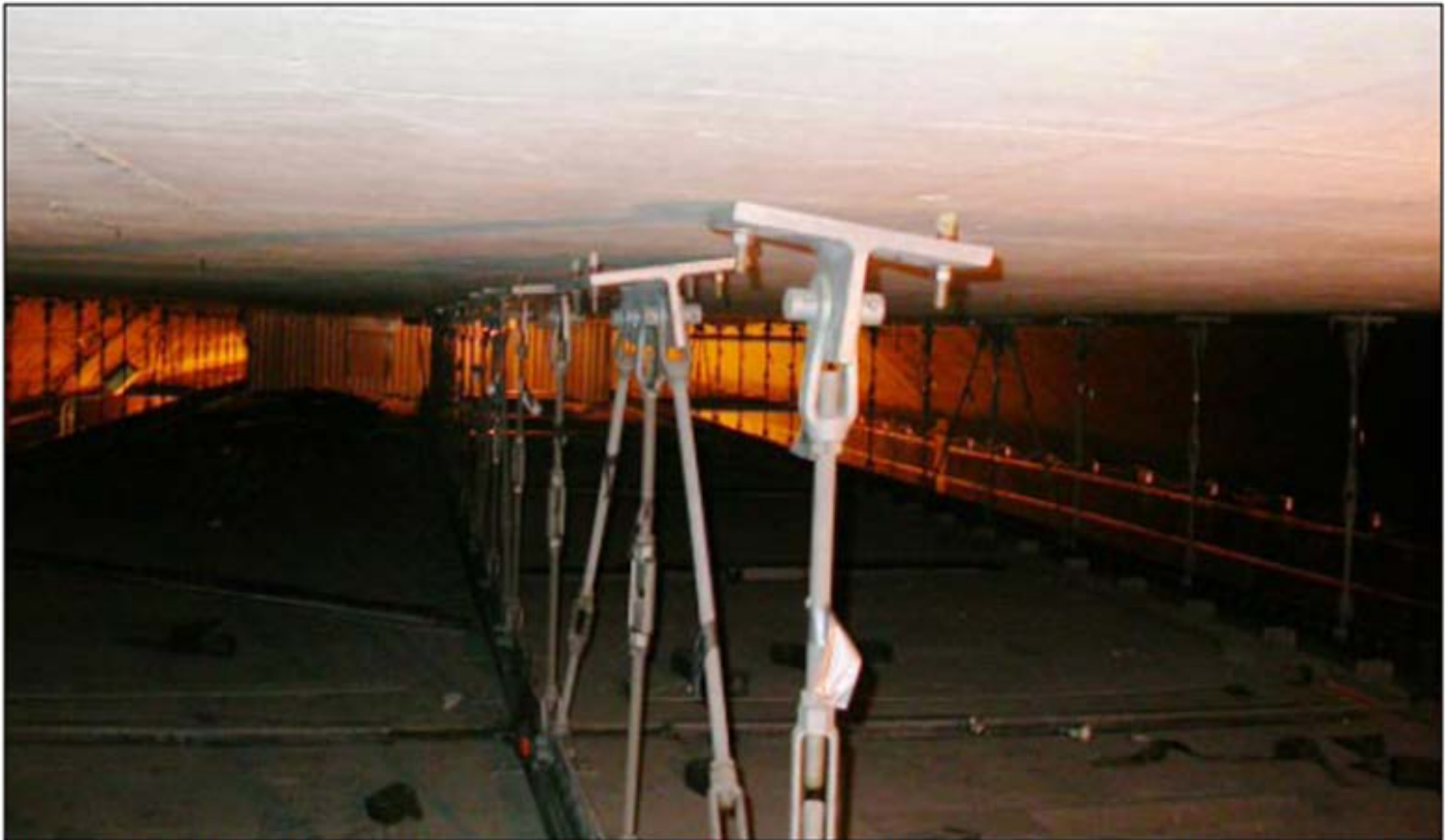
Figure 10. This photograph, taken in the westbound D Street portal tunnel after the accident, shows a number of roof hanger plates that have begun to pull away from the tunnel roof, including the two-anchor hanger plate in the foreground and the four-anchor plate adjacent to it.
