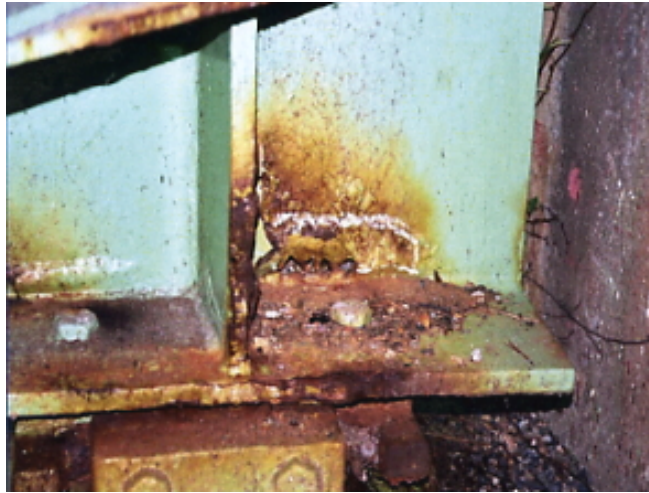
Local corrosion on girder edge
